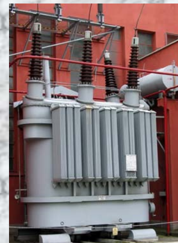
Oil Transformer 16 MVA
